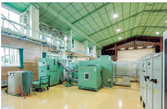
One of the largest motor characteristics testing facilities in Japan *Establishment of Evaluation Laboratory for Next Generation Motors
